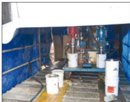
Fig. 10: Plural-component unit staged on scaffolding for on-site application. Photo courtesy of Disnamair S.A.
