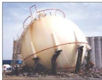
Fig. 11: A sphere collapsed due to undetected corrosion under cementitious PFP. Photo courtesy of International Paint
