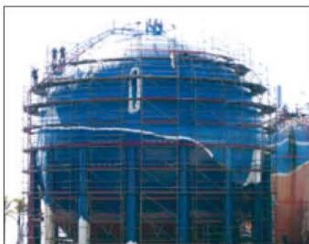
Fig. 9: Coating application on a gas sphere in Tenerife, Spain. Photo courtesy of Disnamair S.A. and Compañía Española de Petróles S.A.
