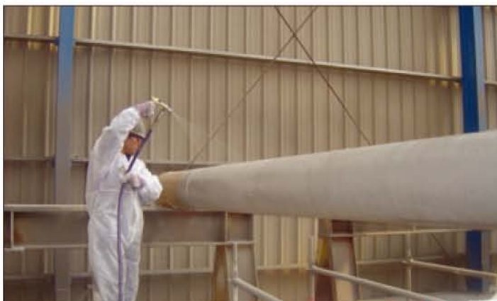
Figs. 5 and 6: Intumescent applied to an offshore platform under construction. Photos courtesy of Disnamair S.A.; WIWA GmbH; and Dragados Off Shore S.A.
